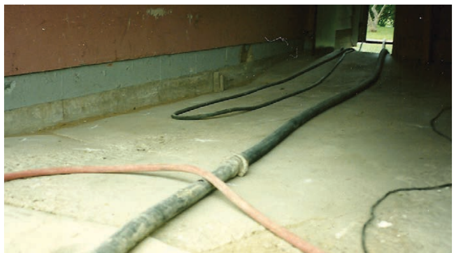
ABOVE: These settlement problems were caused by improper foundation backfill. The walk and garage floor seen here are in the process of being mudjacked back to original elevation.
