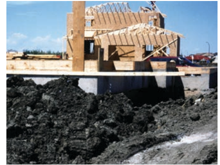
ABOVE: Poorly backfilled foundations using lumps of clay will result in at least 18 inches of grade settlement in the first five to 10 years
